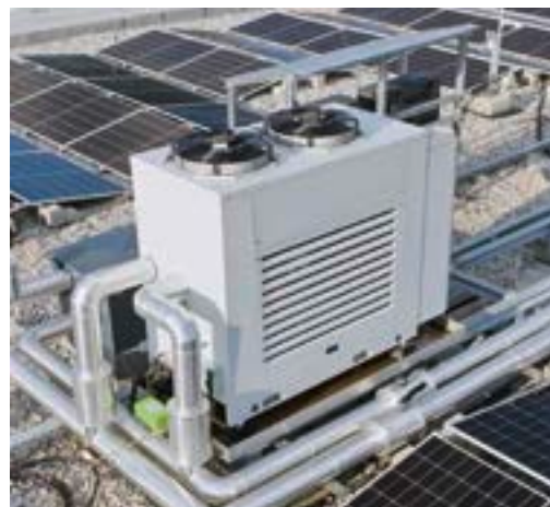
Rittal installed a chiller on the roof, ready to provide emergency cooling.
