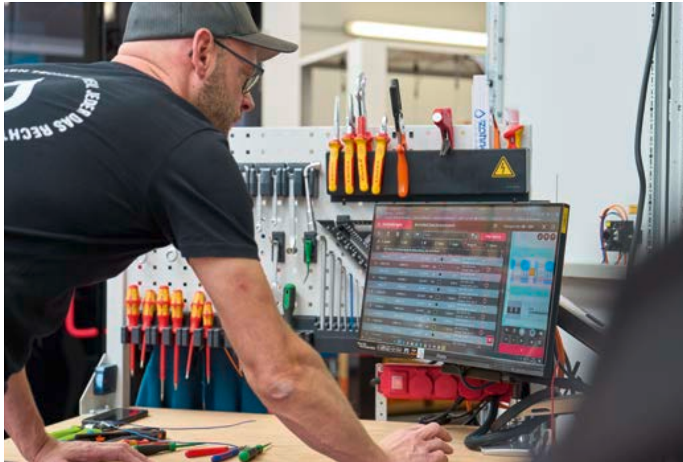
Workers simply need to look at Eplan Smart Mounting to get all the information they need to install components in the enclosure.
