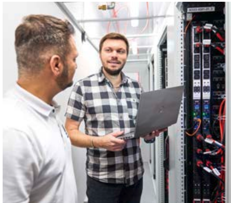
Antonio Giffuni, System Consultant from the Rittal IT field sales team (left) and Christian Dewina in the new BORA data centre.
