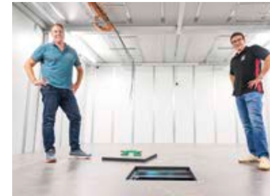
Left: There is a raised floor for climate control purposes. Dr Fiete Dubberke (left) and Michael Nicolai in the Rittal security room, where the next stage will be to install the IT racks.
