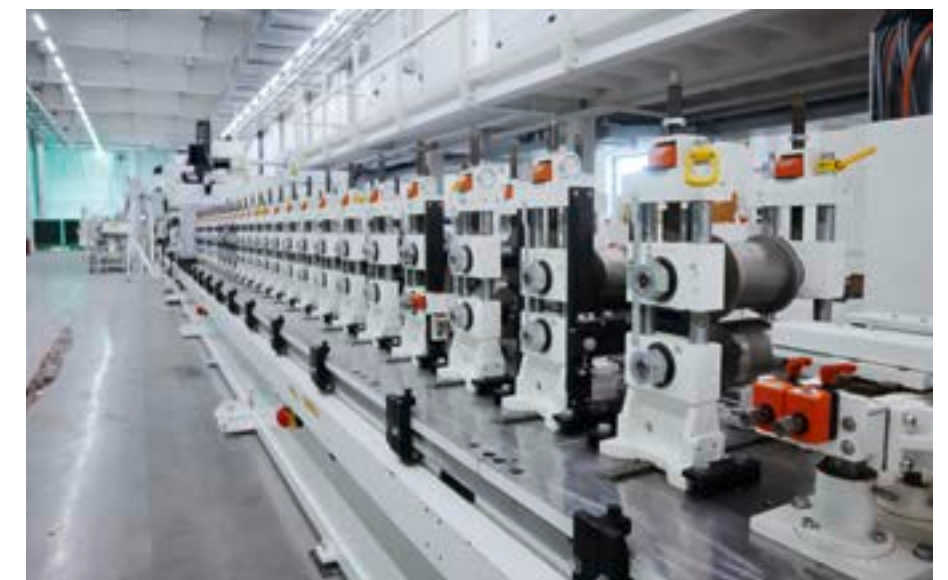
Fast, reliable and efficient: New production lines installed over 10,000 square metres and two floors will continuously boost competitiveness in China.
